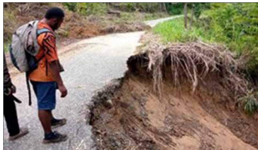
Locals standing on a road which was damaged by a landslide
