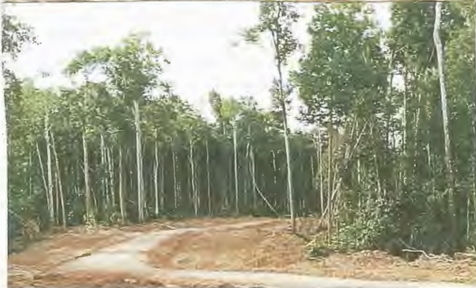
Middle photo - Geo-fabric laid over the treacherous clay followed by corduroy of saplings. Bottom photo - The finished road, after a layer of laterite laid over the corduroy was graded.
